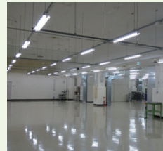
High efficiency lighting equipment
