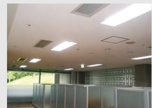
LED lighting in the Industries Development Laboratory
