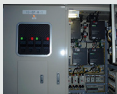
Inverters for air conditioners, exhaust fan, and pumps
