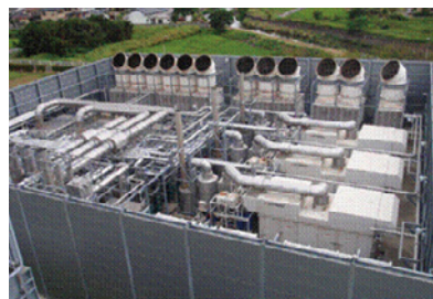
Natural gas cogeneration system
