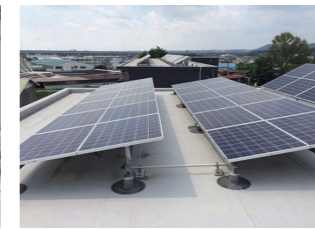
Solar power generation equipment (Nakase company housing)
