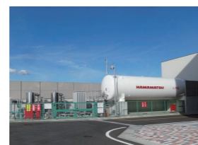
Switch to natural gas
