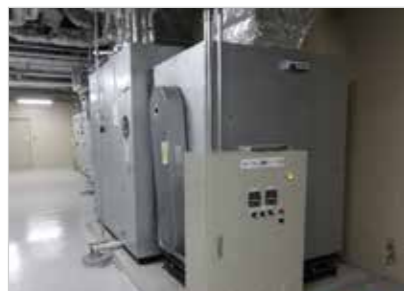
Air handling unit
