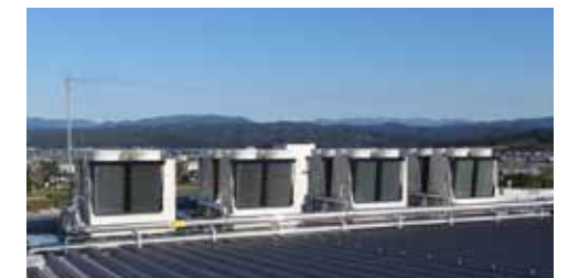
Upgraded HVAC heat sources
