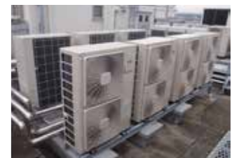
Upgraded HVAC heat source
